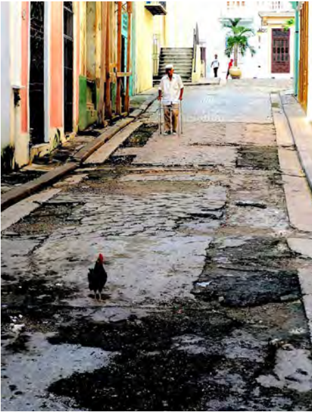
Compared to the situation some 100 years ago, street paving is much better, but maintenance is a serious problem.
