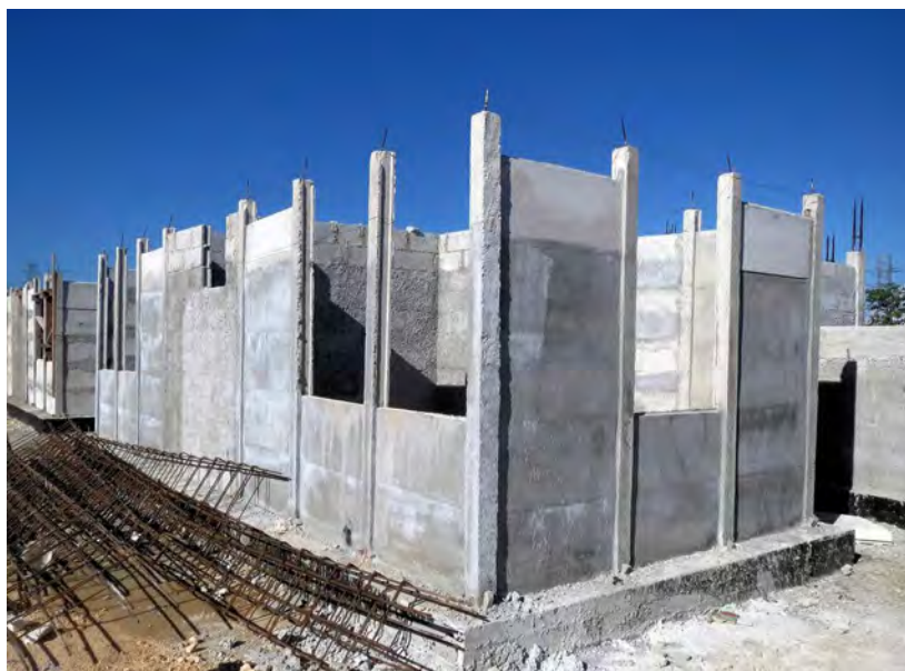
Reconstruction for hurricane victims making use of the Sandino technology in Marianao, 2013
