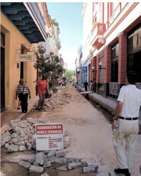
Especially in the historical parts of big cities, Replacement of outdated pipe work in Old Havana, pipework needs to be replaced for health reasons but also to reduce the loss of water due to leakage.
