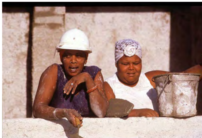
In the microbrigades, women are normal members of the work force. Although many of them are well built, they tend to be given the more delicate jobs like plasterwork or operation of the crane. In social microbrigades they represent the majority of workers.
