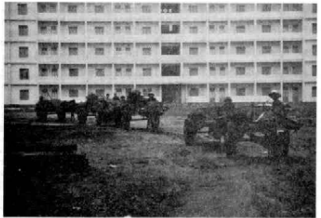
MULTI STOREY HOUSING IS BEING BUILT IN SPITE OF A LACK OF A MODERN EQUIPMENT (Photo: Reuterswård)
