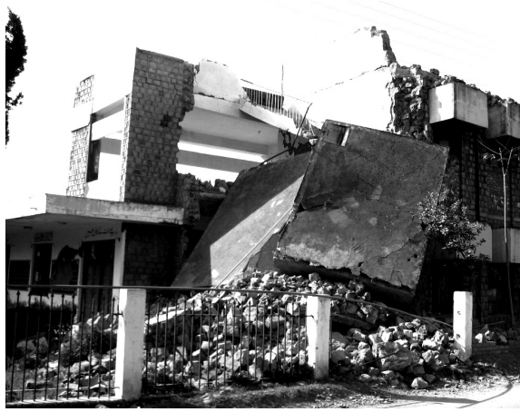
fig 3: The collapsed roof structure of a school in Muzaffarabad, following the October 8, 2005 Pakistan earthquake
