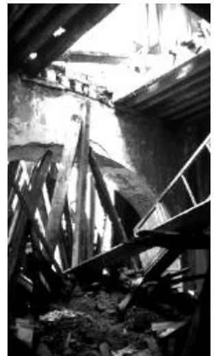
Earthquake damage in a colonial building in the centre of Mexico City Photo: K. Teschner
