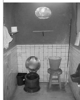
Separating dry installation in residential building in Mexico / Source: S. Esrey, Unicef, New York
