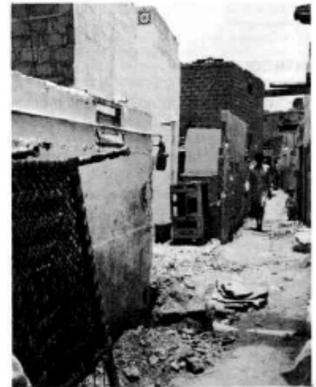
Ghousia Colony: New construction inside the walls of the former houses to make place for the street widening scheme.
