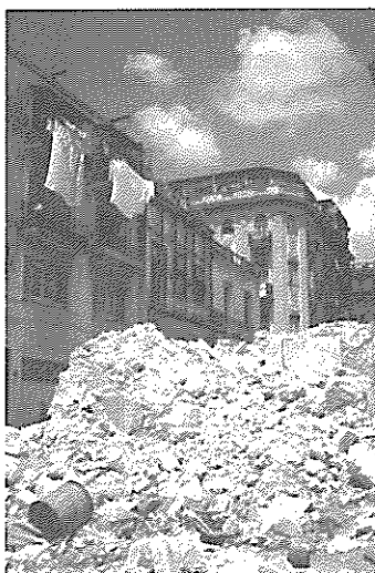
Collapsing houses in Old Havana constitute a health hazard and diminish the stock of historical buildings. (Mathias Pekskamp)
