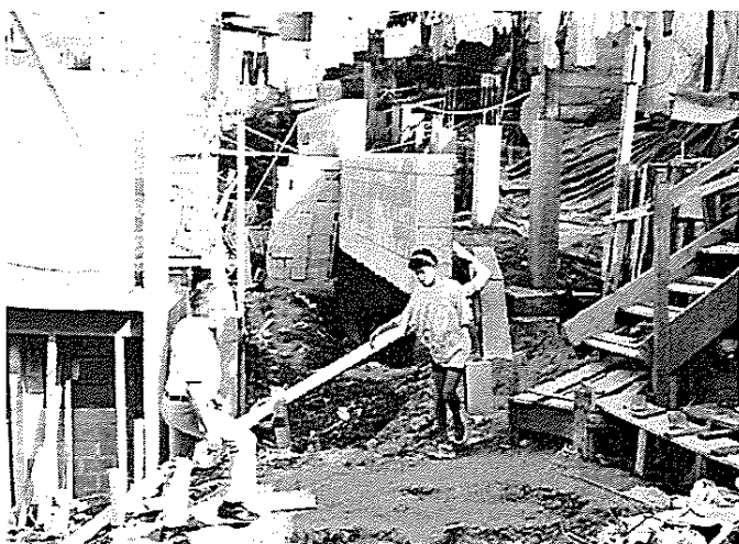
Fig. 1: Upgrading through self-management: construction of a supporting wall and alleys in the favela Sto. Ivo (1991)
