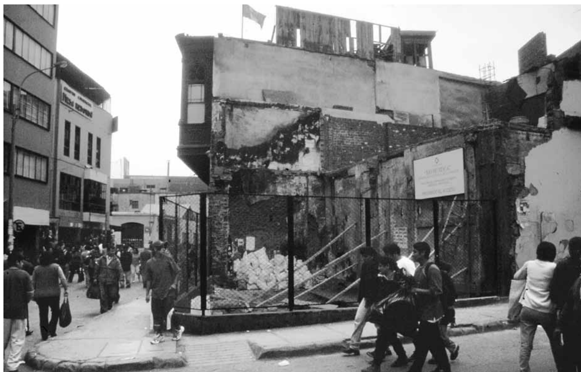
Figure 9-11: Evolution of the corner between Cusco and Andahuaylas streets at Mesa Redonda that was unnoticed by the authorities:
