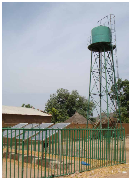
► Figure 2: Solar panel for the health post. Photo: Karin Gaesing
