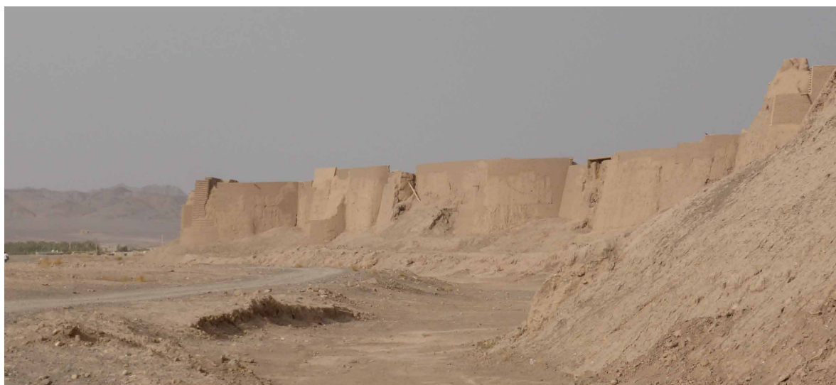
◀ Figure 5: The fortifying wall with the watchtowers of Arg-e Bam. Photo: Renate Bornberg
