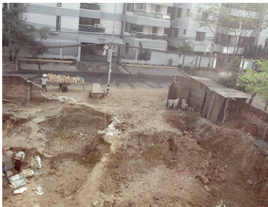
▼ Figure 1: Temporary shelter for construction workers at a building site in Dhaka. Photo: Sabine Baumgart
