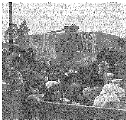
Service supply and standards are not user-oriented ... but here women use the defective water pipes as a collective washing place (Foto: from Mexico; K. Teschner)
