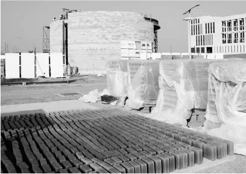
▲ Figure 4: Insulation is a major factor in reducing heat gains. The outer wall of the ECOHAUS is built from light-weight concrete blocks, the core layer is a loose infill of perlite, a granulated volcanic rock. The inner layer is made from compressed earth blocks.
