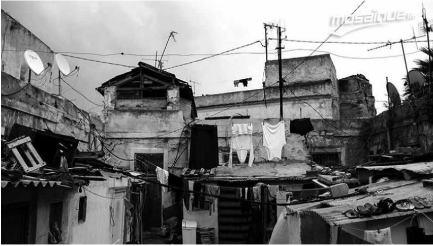
▲ Figure 5: Built environment of one of the Oukalas. Source: Mosaïque FM. Available at: < https://content.mosaiquefm.net/uploads/album/media/thumbnails/147567328444_album.jpg > [last accessed Febr. 5, 2018]
