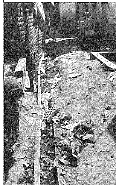
State of negligence before the water and drainage systems started to operate.
