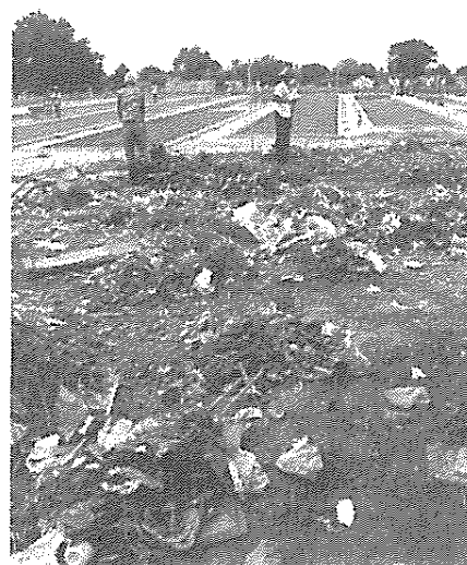
PADE: Biological waste-water treatment and composting of household waste
